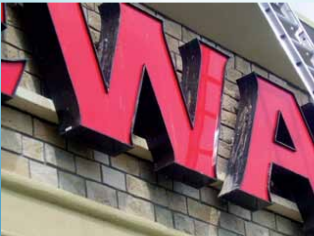
Bird droppings had covered a majority of the shopping centers signs.
