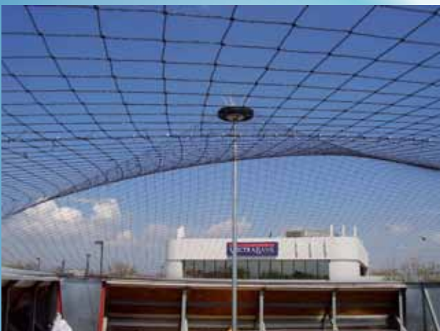
Bird netting installed over the rooftop areas to prevent birds from nesting.
