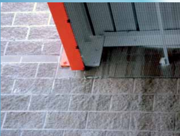
Bird Netting installed under overhangs and eaves to prevent birds from nesting.
