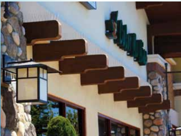
Stainless Steel Bird Spikes were installed over retail entryways to prevent bird mess.
