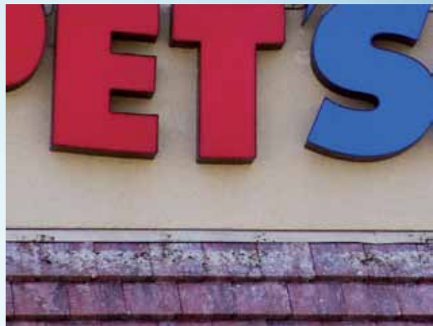
The build up of bird droppings can damage a businesses image.
