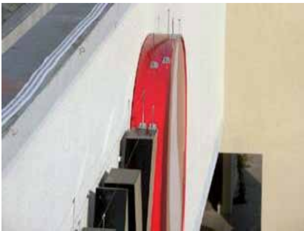
Bird Wire was installed to the tops of the channel letters, glueing the post base in place.
