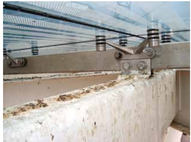
Bird droppings covered the beams and walkways below.
