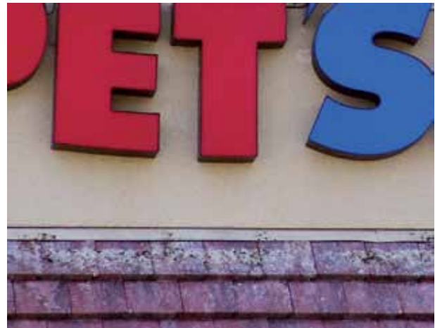
The build up of bird droppings can damage a business's image
