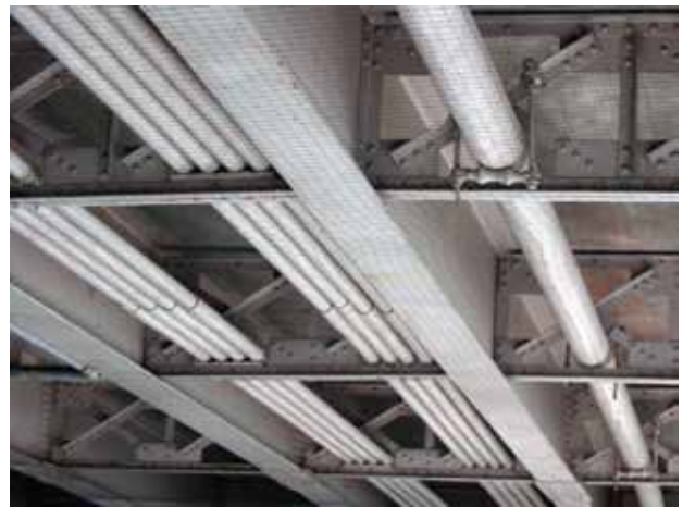
Exposed beams and pipes provided a safe spot for wayward birds.
