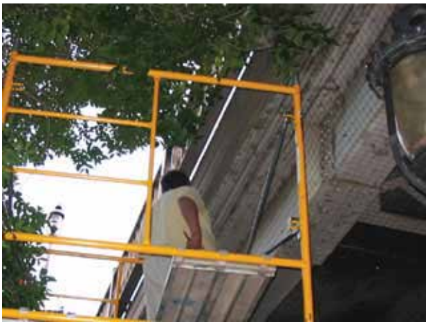
The Bird Netting was installed under and along the sides of the municipal bridge.
