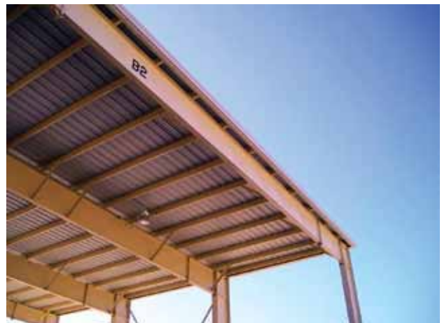
The facility has been bird free, saving maintenance time and money.
