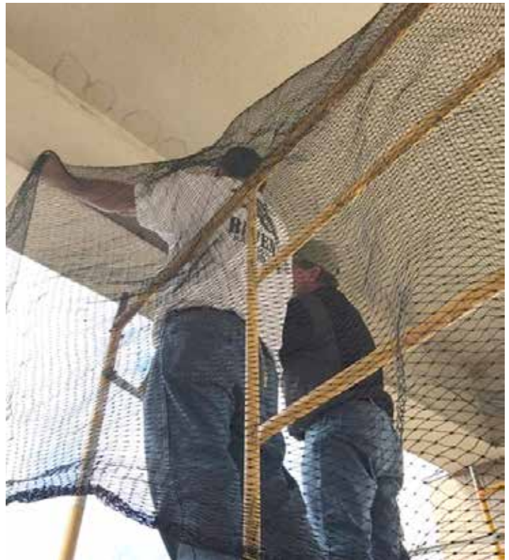
Raven Services installs Heavy Duty Bird Netting to exclude swallows from area.
