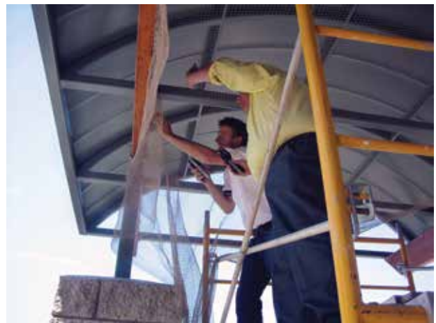
Netting was installed on to the existing wood beams using cable brackets.
