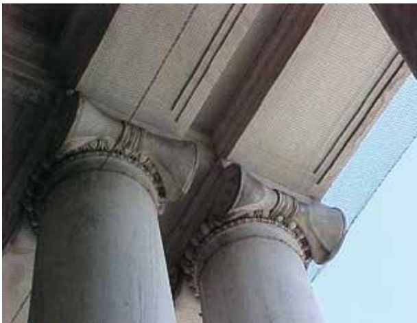
Bird Netting was installed above columns to prevent birds from roosting or nesting.
