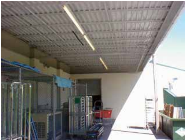
Small birds were nesting in the loading dock area leaving packages and equipment soiled.
