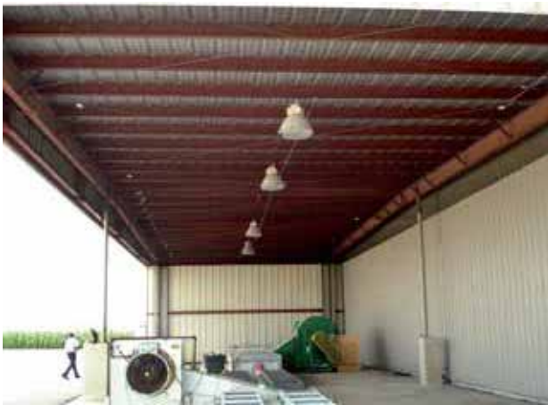
Birds nesting on I-beams were covering storage equipment with bird droppings.
