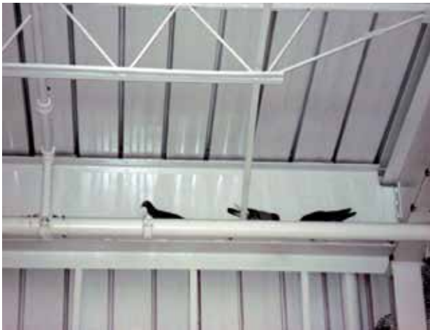
Pigeons were roosting and nesting on exposed beams inside the facility.
