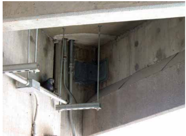
Prior to installation of Bird Slope™, pest birds had complete access to the bridge's ledge.
