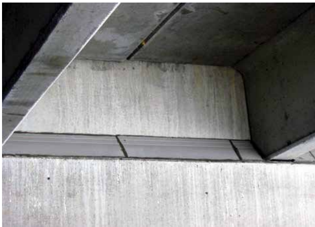
The Bird Slope™ color and dimensions allow it to become virtually invisible on the bridge.
