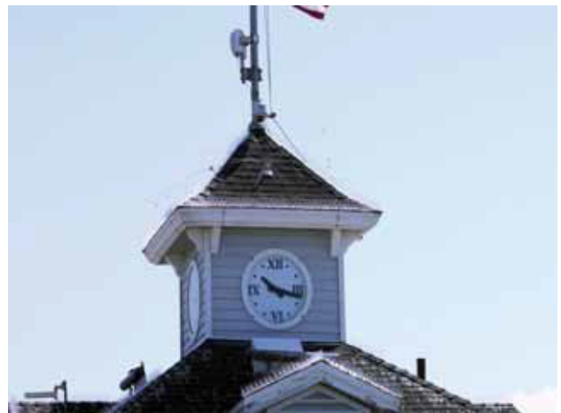
A combination of spikes and bird spiders were used to keep gulls and pigeons off the roof.
