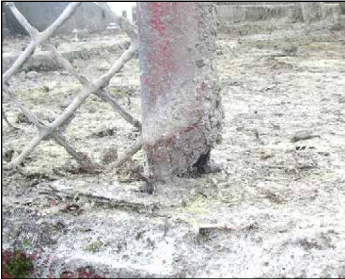
Bird feces corrodes metal post
