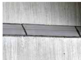
Installed in parking structure
